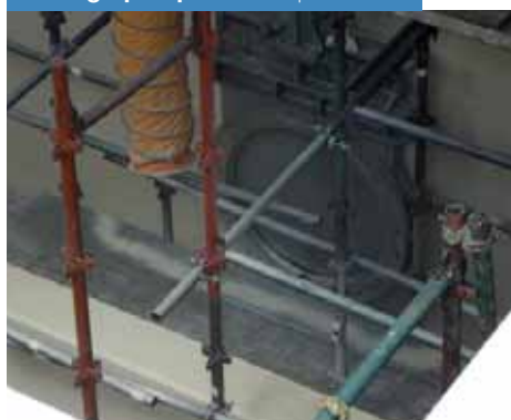
Sewage pump station | Australia
