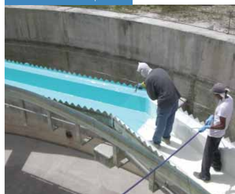
Clarifier tanks | USA
